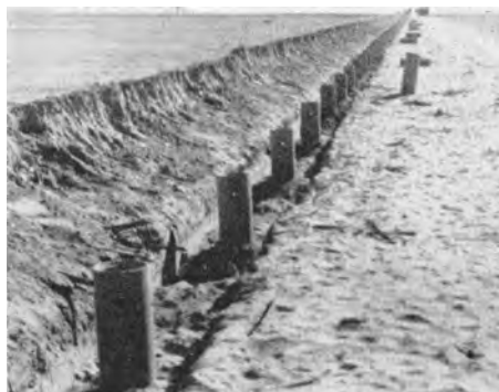
Open pot hydrants being installed for a future vineyard. These hydrants permit small flows in single furrows along each side of the row. The vines will soon require that more soil area be wet. A new water supply is available but it contains almost four times the concentration of salines. The farmer must flood in strips almost 10 feet wide to control salinity. For this, the open pot hydrants are inadequate.
