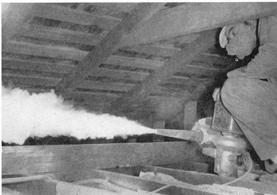
Silica aerogel being blown throughout the attic of a residence from the crawl hole area.
